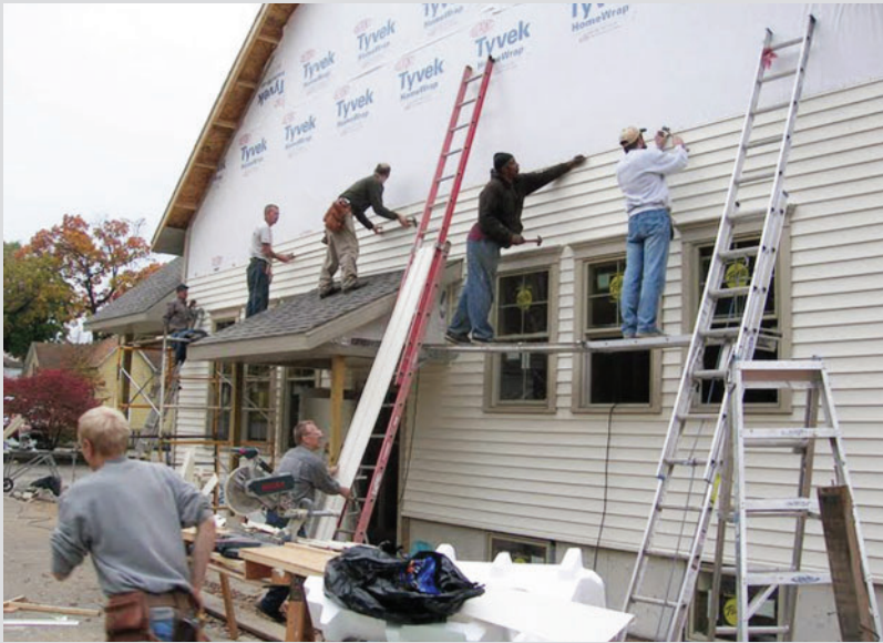
(above, left) During a workday in November 2008, a crew of people from Church Without Walls and Fellowship of Hope and some of FoH's neighbors install siding on the addition. (above, right) Jonathan Fridley of FoH and neighbor David Fayne enjoy a break from their work. (Photos provided by Verlin Miller)
